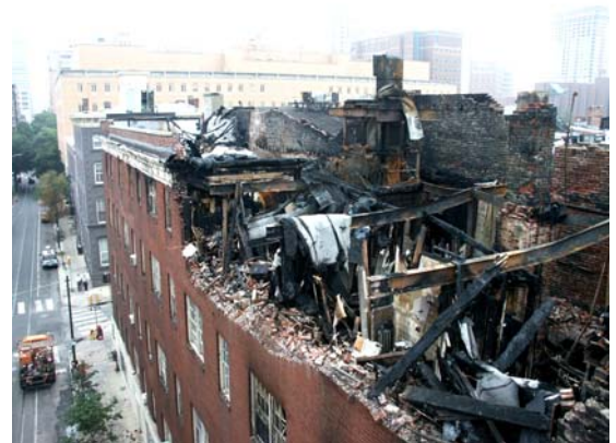
Fire Damage taken by one of our engineers from a crane boom.
