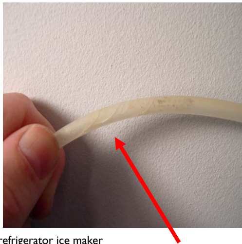
Photo 2 – Failed water supply line for an refrigerator ice maker
